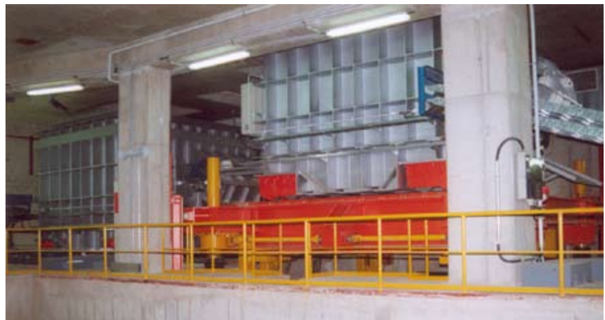
Figure 1. The melting pots in their operating position one story below the production line
